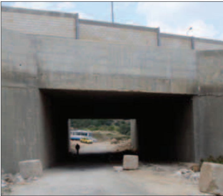
A new road for settlers above — a tunnel beneath it for Palestinians
